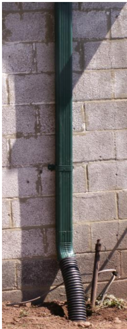
Gutters and downspouts can control and direct rainwater from our roofs
