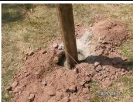
Where necessary the post holes were dug and concrete was used to add stability
