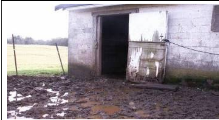
"Before" the bluestone paddock was installed water pooled in front of the stall.
