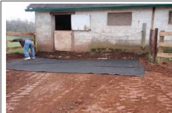
We used a felt-like material called filter fabric in front of the barn that will allow rainwater to soak through but will keep the soil from rising up and mixing with the bluestone.
