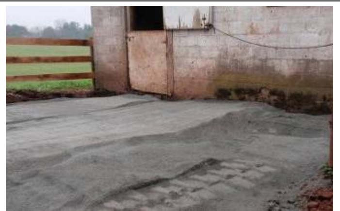
Bluestone dust was placed on top of the filter fabric, level with the door to the stall.
