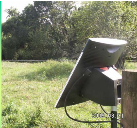
Gallagher Solar Charger (Back Field)
